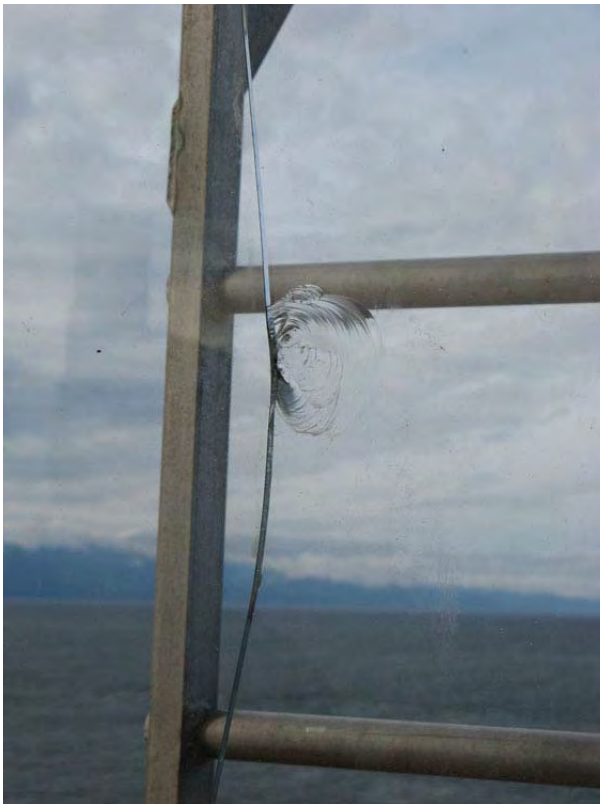
Figure 34: Vertical crack in the west pane of glass. (HCN/2007)
