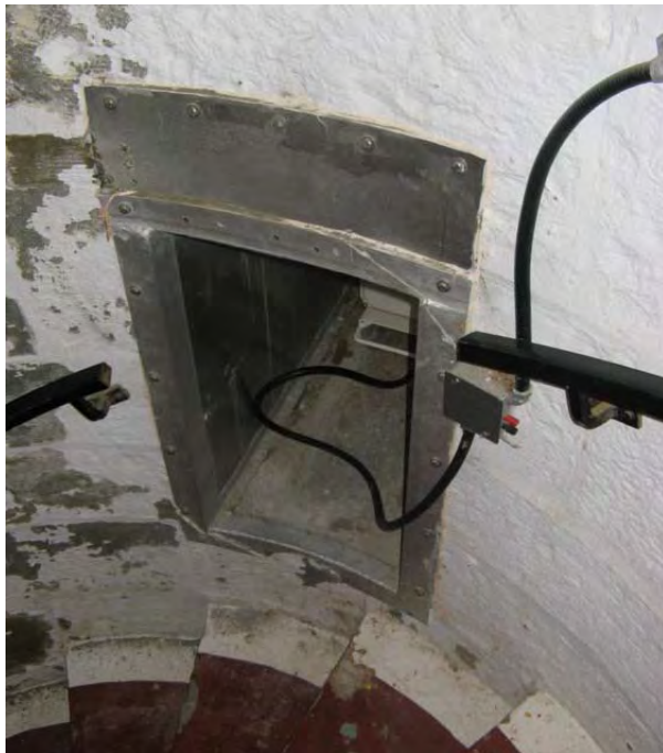
Figure 52: Interior side of the second opening from the top, fitted with the fog-detector. (HCN/2007)
