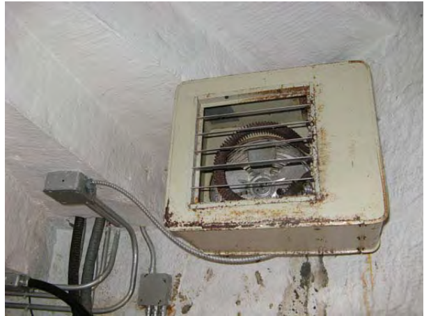
Figure 49: Electrical heater, now out of use. (HCN/2007)
