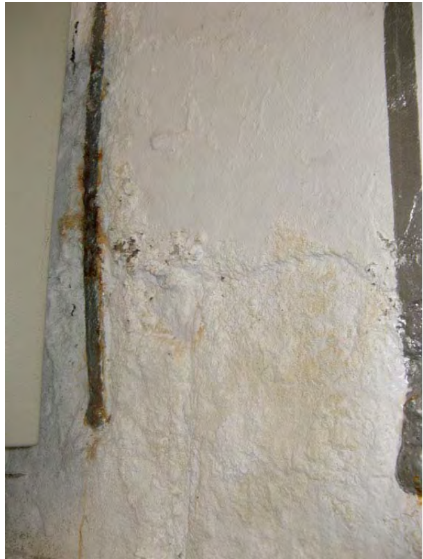
Figure 25: Corroded metal ties at the top of the interior walls. (HCN/2007)
