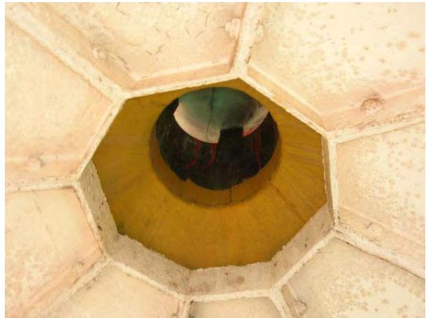
Figure 33: Underside of the lantern cupola and mildew stains. (HCN/2007)
