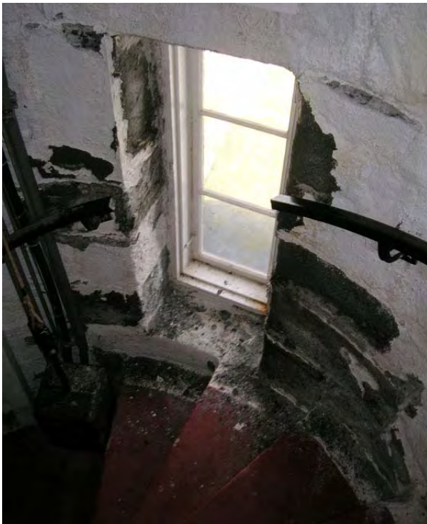
Figure 22: Stone deterioration around the interior of the top window opening. (HCN/2007)
