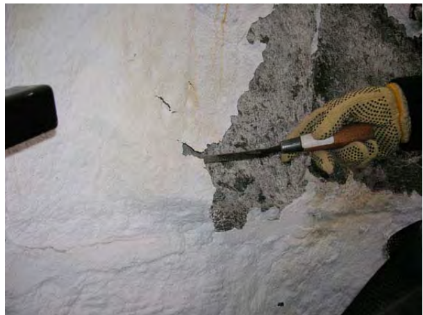
Figure 23: Paint failure on the interior face of the walls. (HCN/2007)
