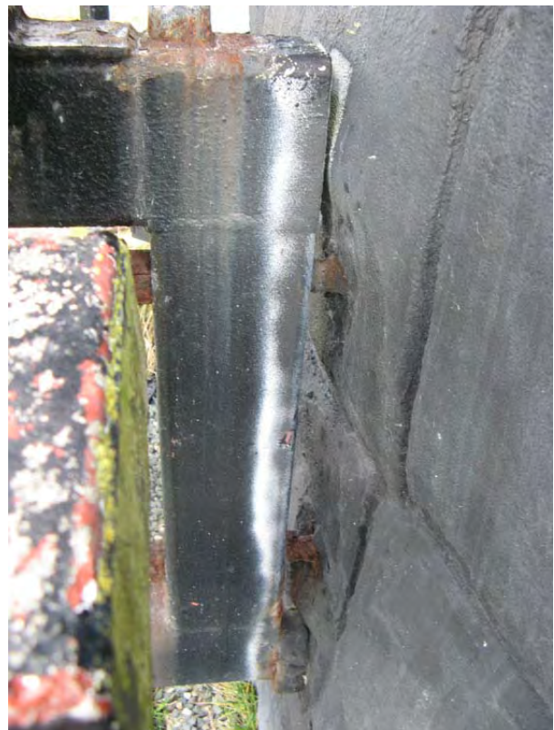
Figure 59: Stair brackets and corroded anchors set into the stone wall. (HCN/2007)
