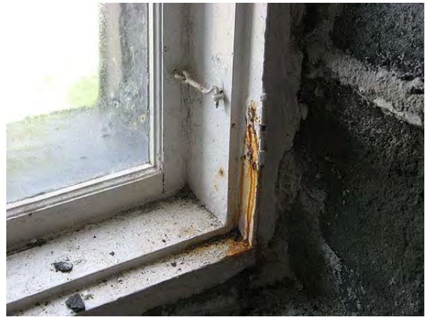
Figure 51: Typical deterioration of the wood sash: corroded metal hooks, staining and stone damage concentrated at the base of the opening. (HCN/2007)
