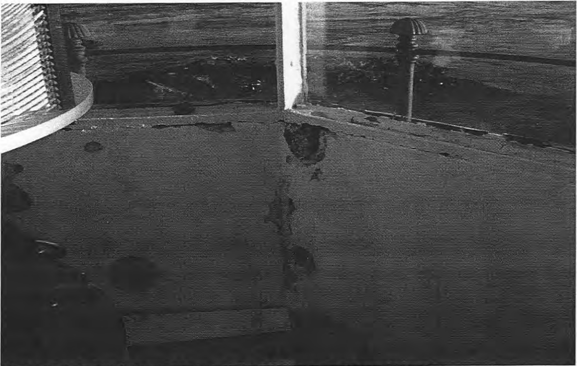
Photo 3. Interior of Lamphouse showing deteriorated concrete.
