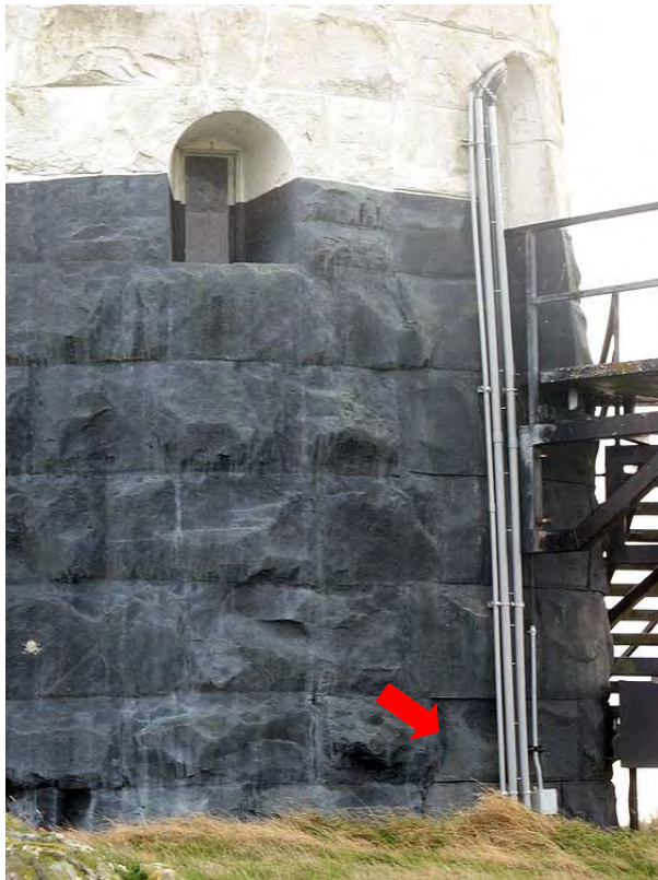
Figure 12: Large hammer-dressed coursings of the tower foundations, below the door opening. Note the transition from parging to natural stone right of the door opening, next to the conduits and the vertical crack along it. (HCN/2007)
