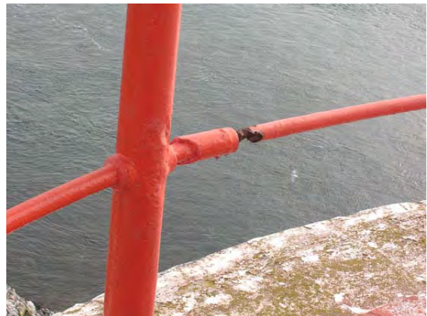
Figure 47: Corroded guardrail. (HCN/2007)
