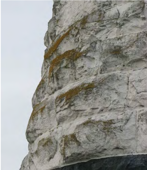
Figure 20: Algae growth on the south face of the tower. (HCN/2007)
