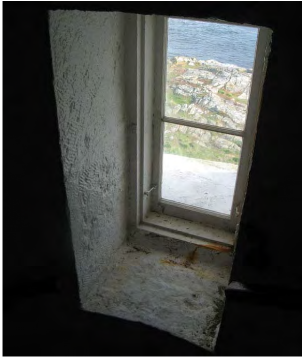
Figure 50: Window opening at the base of the tower and its wood sash. (HCN/2007)
