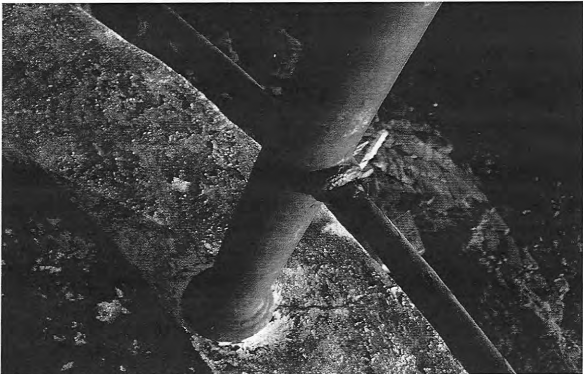
Photograph 5. Deck of Lamphouse showing Peeling Membrane.
