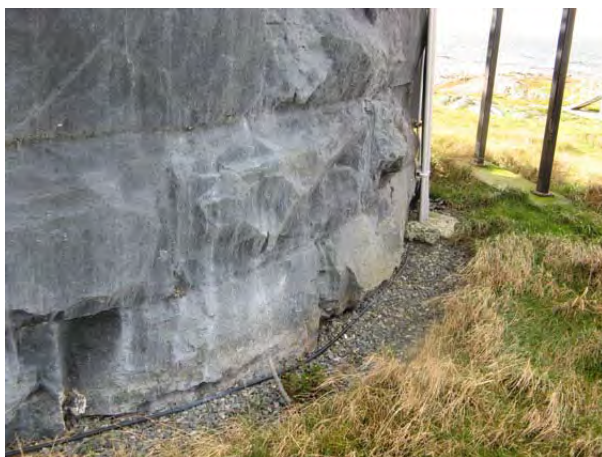
Figure 14: Breaks in the base course and white streaking. (HCN/2007)
