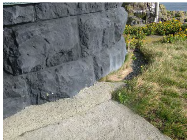
Figure 15: Asphalt surface abutting directly against the base of the tower. (HCN/2007)
