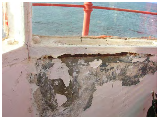
Figure 39: Corrosion and paint failure on the interior face of the parapet. (HCN/2007)
