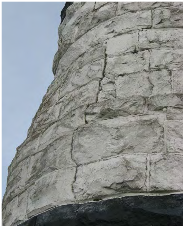
Figure 18: Vertical crack extending along the southwest face of the tower. (HCN/2007)
