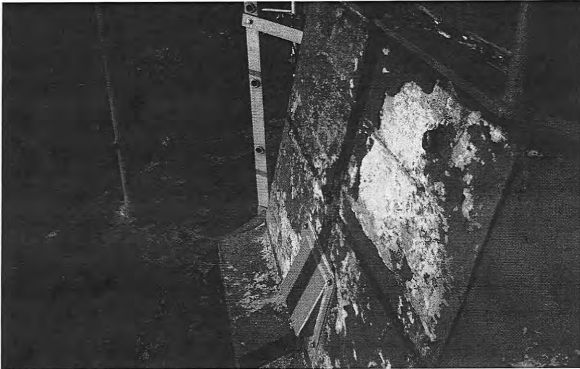
Photograph 4. Exterior of Lamphouse showing Peeling Paint.
