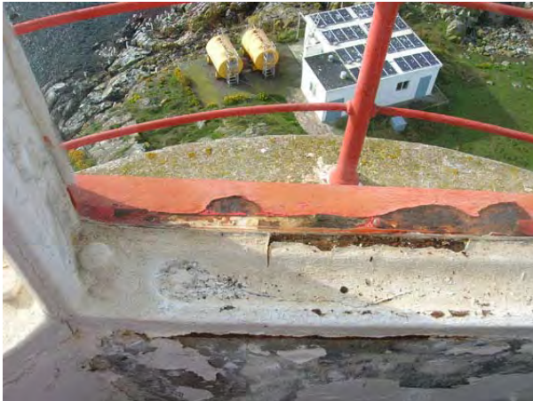
Figure 36: Corrosion and rotted exterior wood stops along the outer sill of a storm panel. (HCN/2007)
