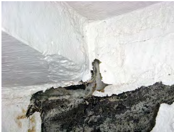
Figure 26: Traces of deterioration at the junction between the stone steps and the tower walls. (HCN/2007)
