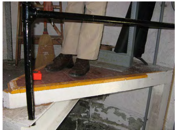
Figure 29: Concrete landing and wood platform at the top of the spiral stair. (HCN/2007)
