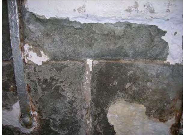
Figure 21: Delamination of the stone on the interior face of the top walls. (HCN/2007)
