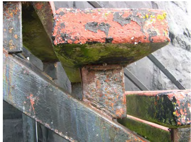
Figure 57: Surface corrosion on the structural members. (HCN/2007)
