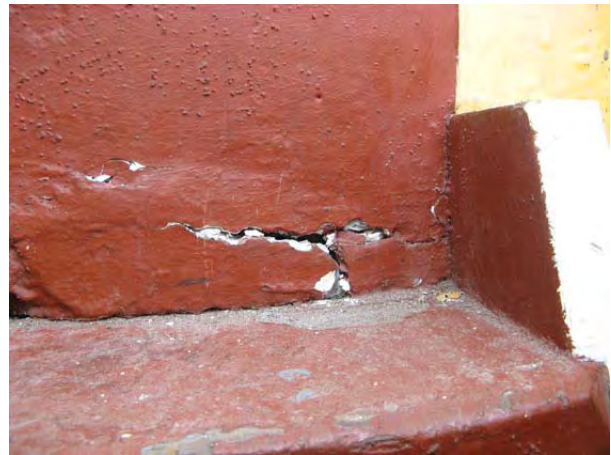
Figure 31: Deterioration of the concrete slab at its connection to the ladder. (HCN/2007)
