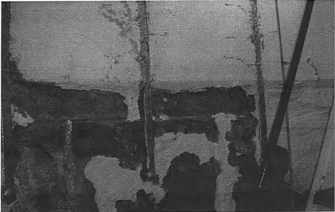
Photo 2. Scaling of Interior Sandstone.
