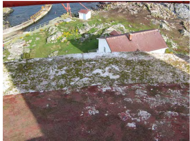
Figure 45: Coating failure and hairline cracks on the gallery. (HCN/2007)
