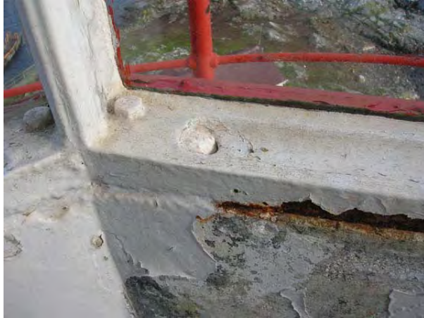
Figure 40: Condensation gutter and obstructed drain. (HCN/2007)
