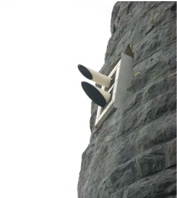
Figure 53: Exterior view of the fog-detector and the broken stone lintel above it. (HCN/2007)
