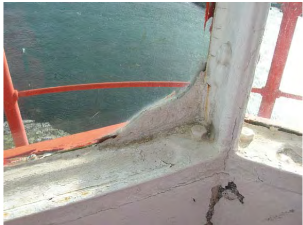
Figure 35: Large amount of caulking concentrated in the lower corner of a storm panel. (HCN/2007)
