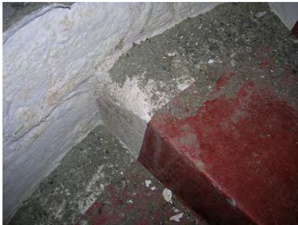
Figure 24: Debris accumulation on the steps. (HCN/2007)
