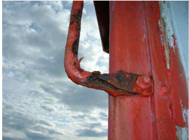
Figure 37: Corroded exterior hand-hold. (HCN/2007)
