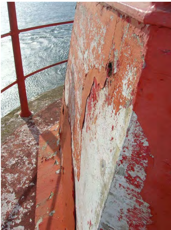
Figure 38: Exterior paint failure on the concrete parapet. (HCN/2007)
