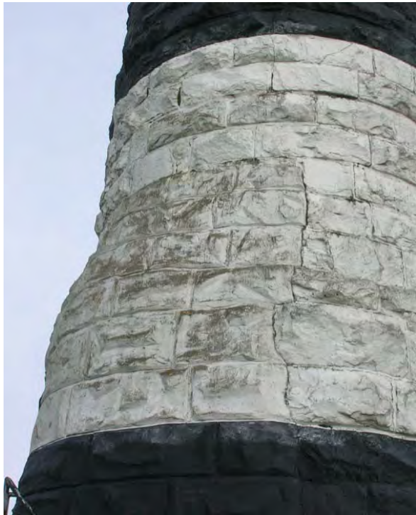
Figure 16: Deformed exterior tower wall at its former point of connection with the demolished residence. (HCN/2007)
